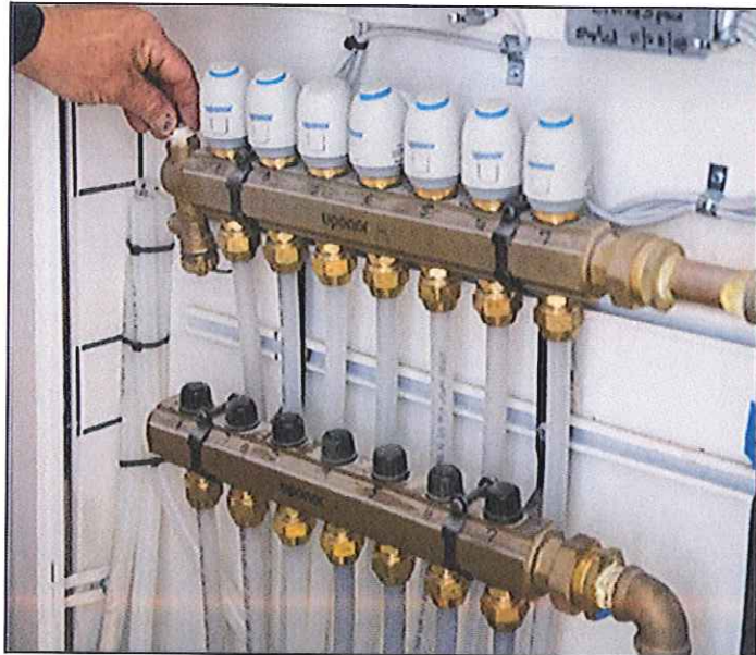
In addition to the 18,500 feet of Uponor PEX tubing for the radiant and snow-melting systems, the Wormley Row restoration also featured 14 Uponor TruFLOW™ manifolds.
